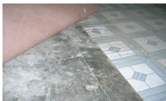
Fig. 1: Mold and fungal spores below the vinyl floorings
