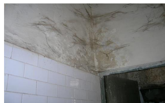
Fig. 3: Fungal spores ideally grown at unattended toilets side needs attention
