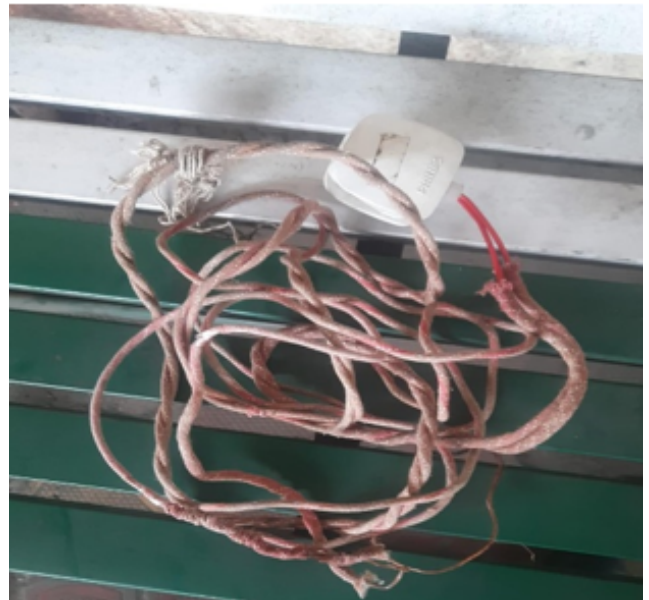
Fig. 2: Photo of disconnected electric wire having uninsulated ends.
