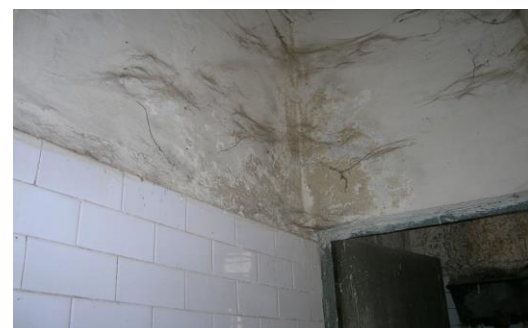
Fig. 3: Fungal spores ideally grown at unattended toilets side needs attention
