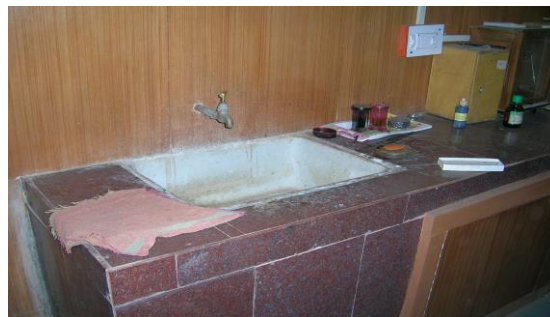
Fig. 8: Wooden material contains biological material provides place for fungi and molds.
